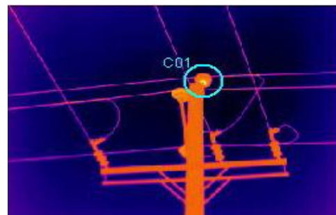
Figure3. An example of IR defect detection of in-service insulators
